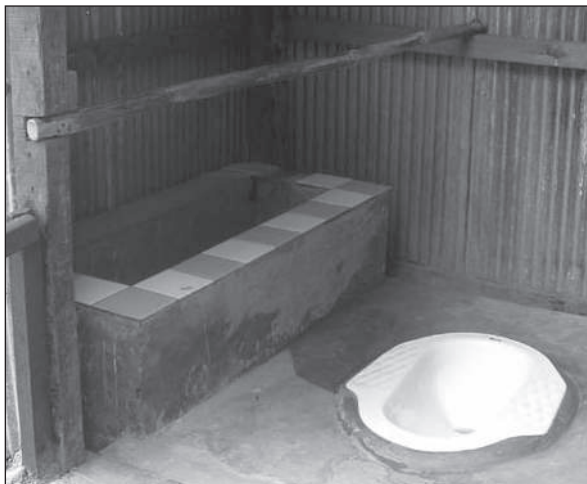
Figure 7.53. Water trough inside toilet cubicle. (Case-study 9.19, page 215)
