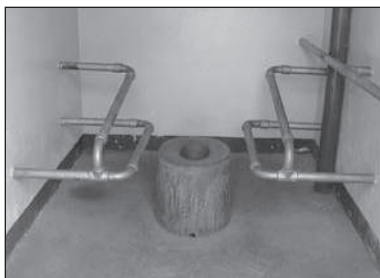
Figure 9.124. Raised toilet seat with handrails for support.
