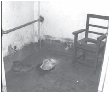
Figure 9.18. Multi-purpose bathroom with toilet in corner.
